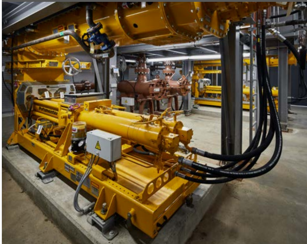
KOS high density solids pump with S-tube technology under crane drop bunker
